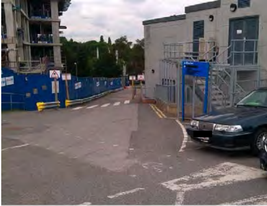
View from outpatient's car park towards the existing theatre block and phase 2a building
